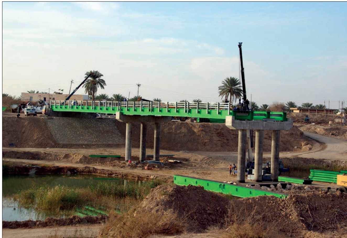
A Unibridge® road solution built in Bagdad in 2010. The Unibridge® Mining Solution will use the same principle for the abutments and piers.
